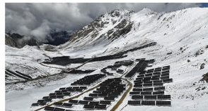
Phase I of Nagu Solar Power Station
