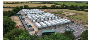
Minety Battery Storage
